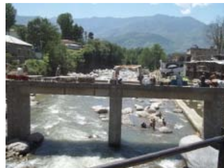
Newly constructed bridge after destructive floods in Batagram district (Photo by Waqar Tareen)
