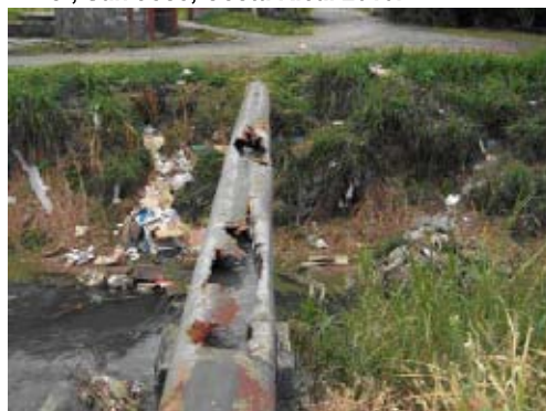
Picture 1: Sanitation infrastructure at the Tiribí River, San José, Costa Rica. 2010.
