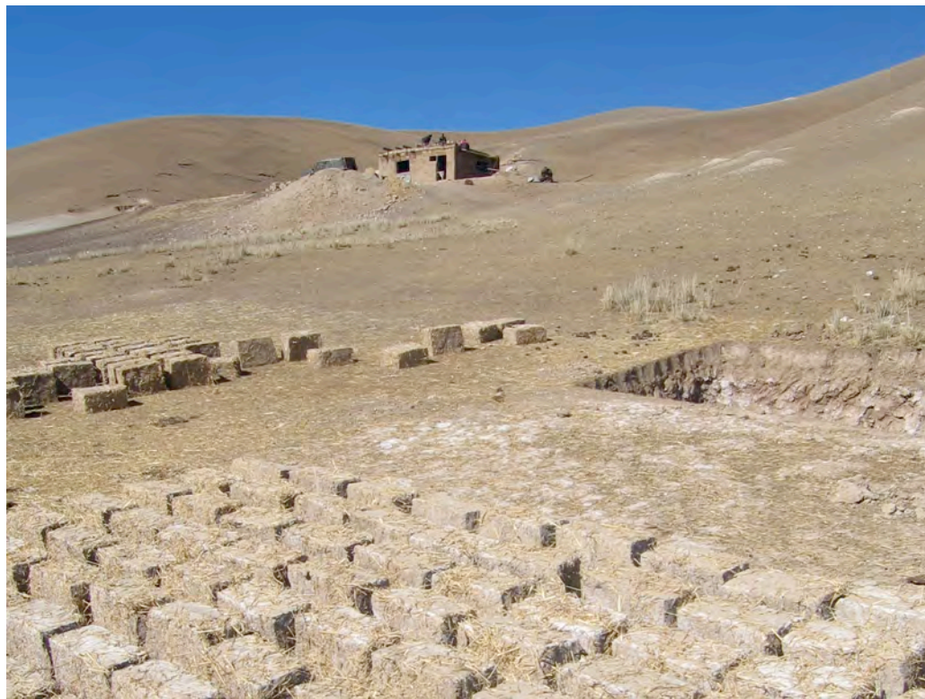
Figure 10.3 Construction of a new saray on the intensive pastures of Botosh, Kyzyl-Tuu (photo by the author, 2007)
