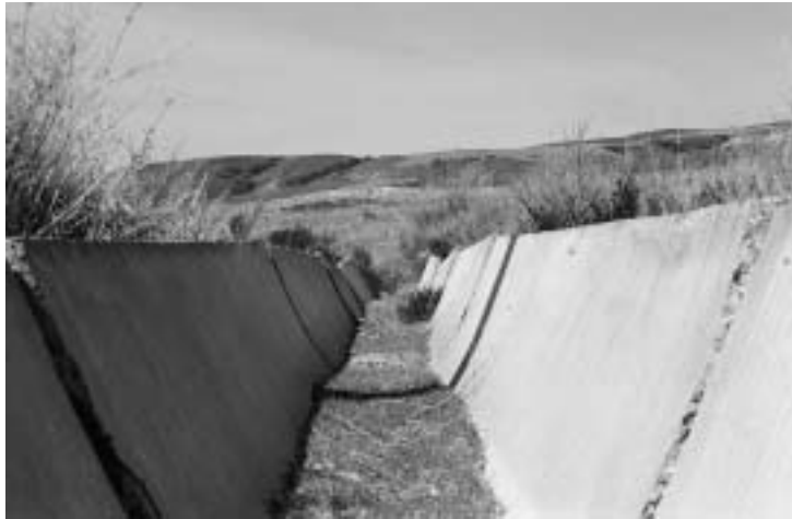
Fig. 5 Irrigation is of vital economic importance in the semi-arid zones of Central Asia, provided that infrastructure is maintained. Photo: Brigitte Portner, July 2001
