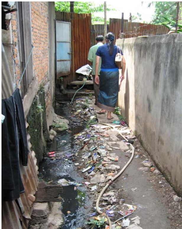
Figure 2.3: Rudimentary open drainage, solid waste dumping. (Photo: Sandec)
