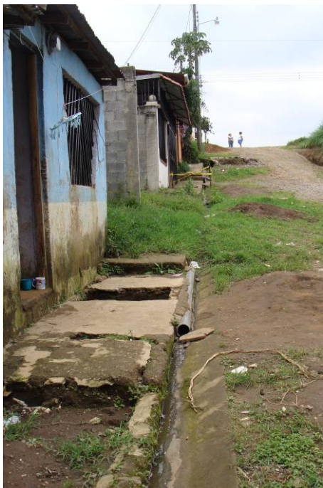
Figure 5.6: Greywater discharge into a street. (Photo: Sandec)
