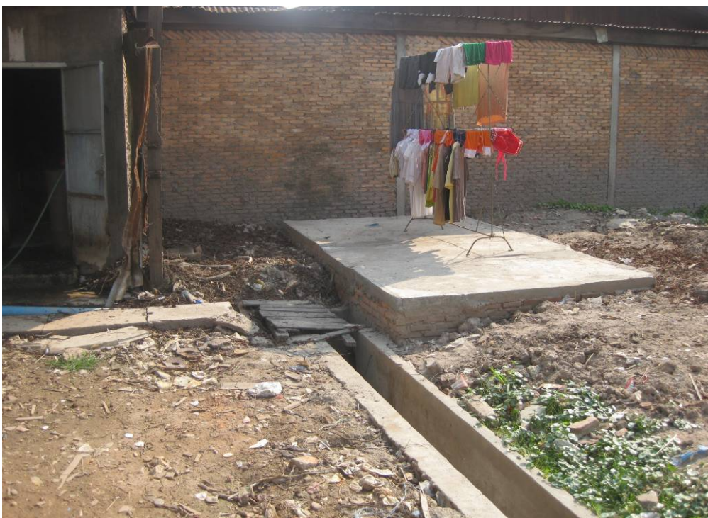
Figure 2.10: Community septic tank treating the wastewater of 20 households. (Photo: PTI)
