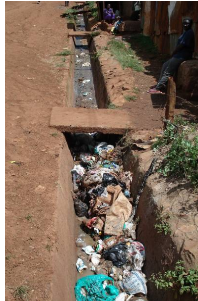
Figure 3.6: Stormwater drains with solid waste in Waruku. (Photo: Sandec)
