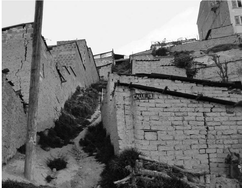
Fig. 3 Damaged homes in La Paz. (Photo by Fabien Nathan)
