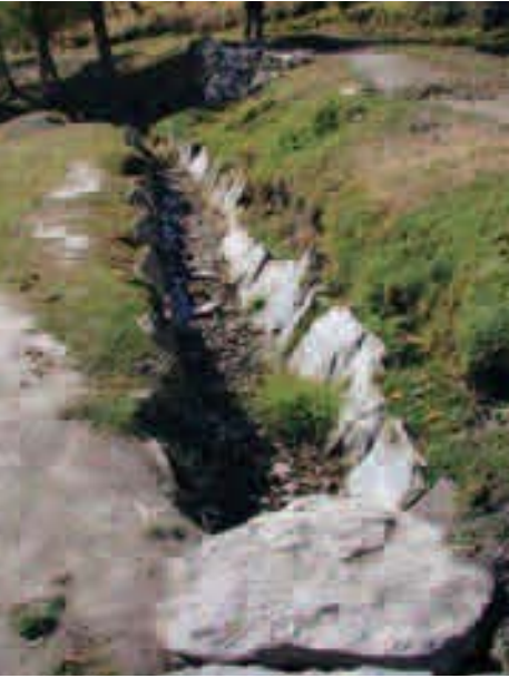
Proper planning and regular maintenance of irrigation systems are labour-intensive. Inappropriate schemes can lead to declining soil fertility, while leaking irrigation channels can trigger mudflows. (Photo: J. Schneider)
